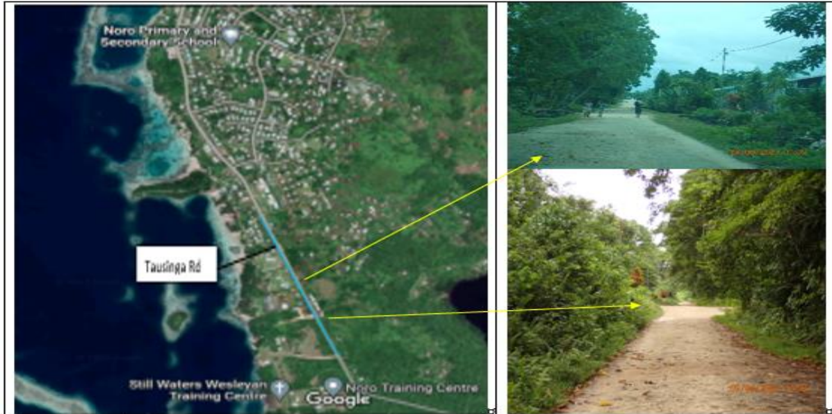
Figure 5: Tausinga road condition
