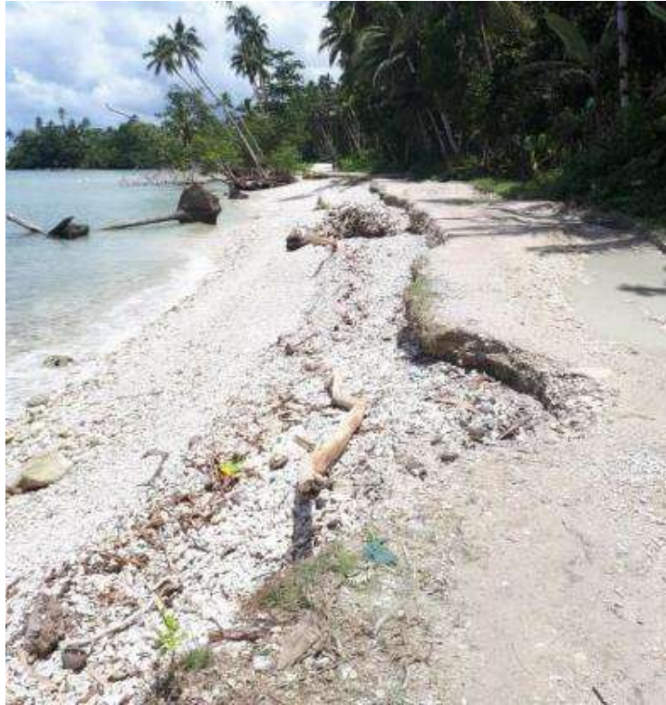
Figure 11: Road erosion along coastline on northern road
