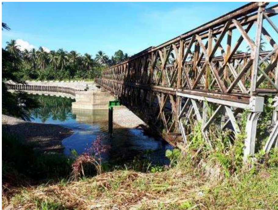
Figure 12: Fiu Bridge close to Auki which has been identified for upgrading under SIRAP
