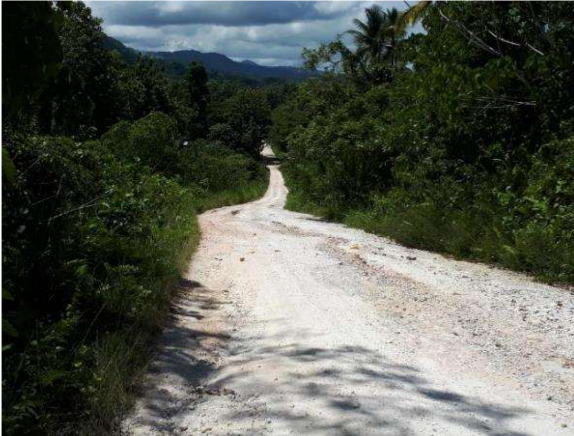
Figure 14: Steep section on southern road showing signs of run off and gullies.
