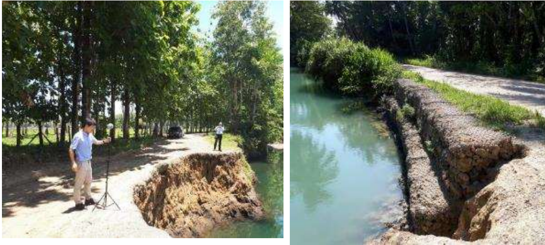
Figure 20: River bank and road scour at Bina (l) and Dala (r).
